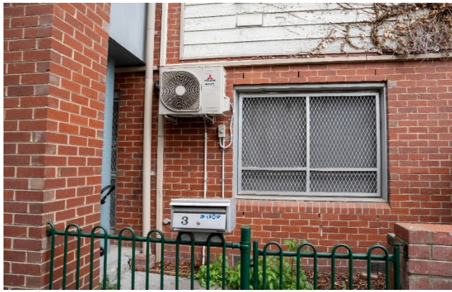
Credit: Homes Victoria, Split System Heating and Cooling, Campbell St Collingwood
